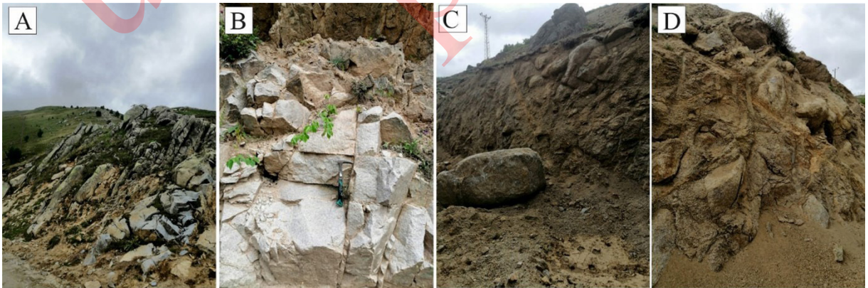
Figure 3- a-b) Cracking systems in the rocks of the Kazıkbeli Pluton, c-d) Arena formation observed in the rocks of the Kazıkbeli Pluton.
